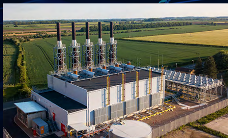
HiIROC 'Gas peaking' plant
